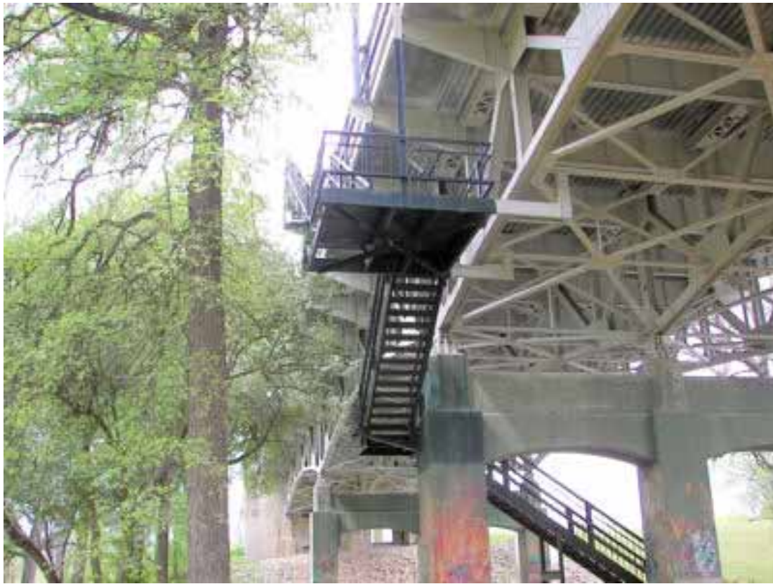
This platform which is 24'8" from the ground makes a great rigging point for vertical practice.
